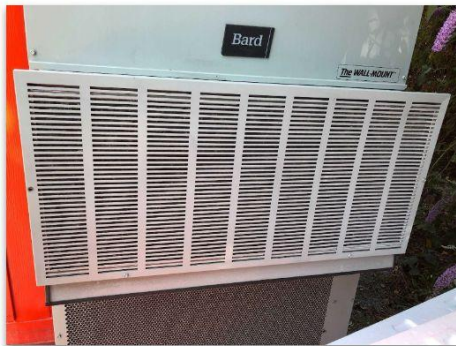
Replace Bard HVAC air filter
